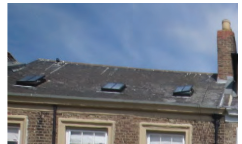
Although small, these rooflights are very noticeable and disrupt the flow of the roofscape
