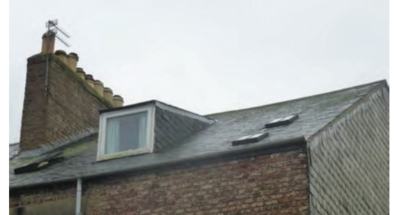
Catslide dormers are visible on the rear slopes of Northumberland Square (east side)
