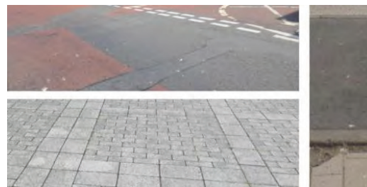
Inconsistent standards of road and footpath surfacing
