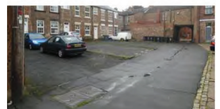
Missing yard walls expose rear elevations and allow back yards to 'bleed' into back lanes, creating large unattractive spaces
