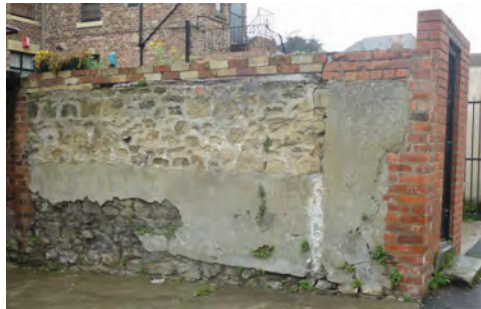
Unsuitable materials have been used to repair walls, causing damage to historic fabric
