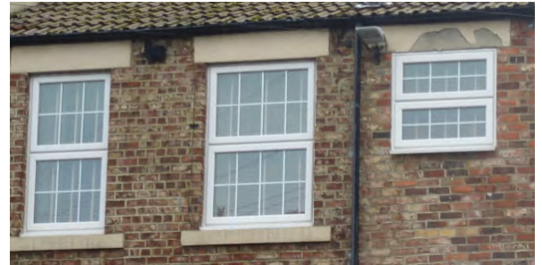
The installation of PVCu windows to this property has altered the appearance of the building, with flat, flimsy glazing bars and too chunky frames
