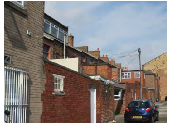
Patched masonry and render, altered yard walls and offshots, Howard Street east
