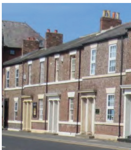
Paired Tyneside flat doorways, simple sandstone surrounds and steps, Upper Norfolk Street
