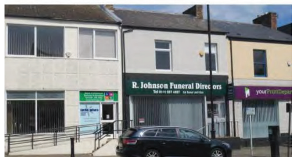
Widened window openings and inserted shopfronts. PVCu windows have also been set flush with the buildings face.
