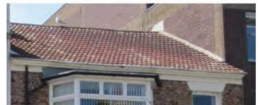
Render, cladding and painted sandstone conceal historic shopfronts. Concrete tile roofs are also at odds with traditional slate.
